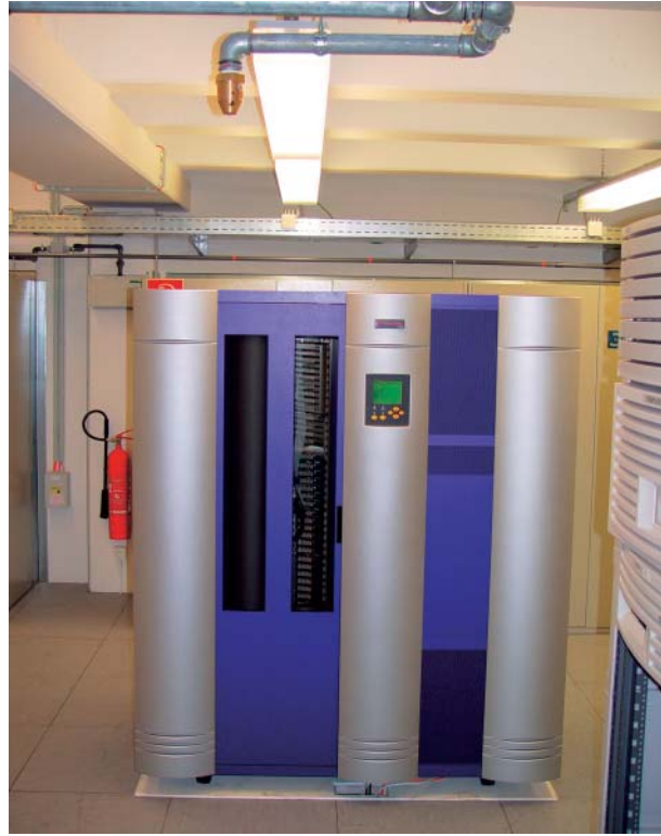
Protected EDP room
