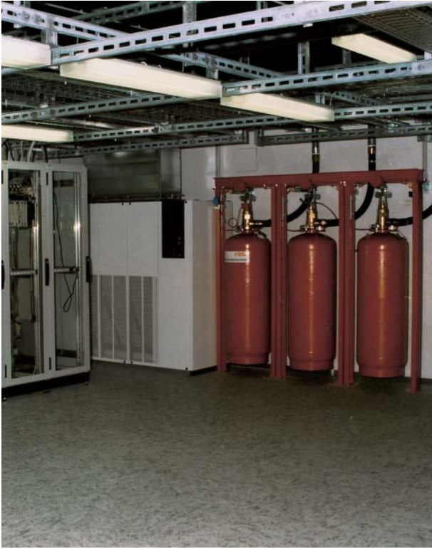
KD-200 system for an EDP room
